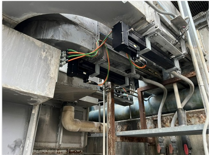
Figure 3. Electronic diversion gate at Lower Granite Dam.
