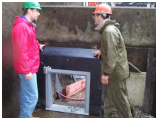
PTAGIS Software Engineer John Tenney (l) and NMFS Biologist Earl Prentice (r) discuss the installation of an evaluation PIT tag interrogation tunnel in the adult fish ladder at Bonneville Dam.
